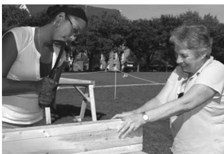
URI women studies major Celandra Montilla hammers nails into lumber while communications studies professor Lynne Derbyshire holds the two-by-fours steady. The Habitat for Humanity “House in a Box” was delivered to the gulf area in November. Photo by Nora Lewis, courtesy of URI.
